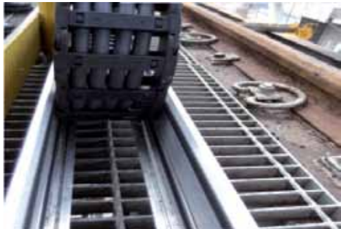
China Steel Corporation, Yenhung Lin, Kaohsiung City, Taiwan
